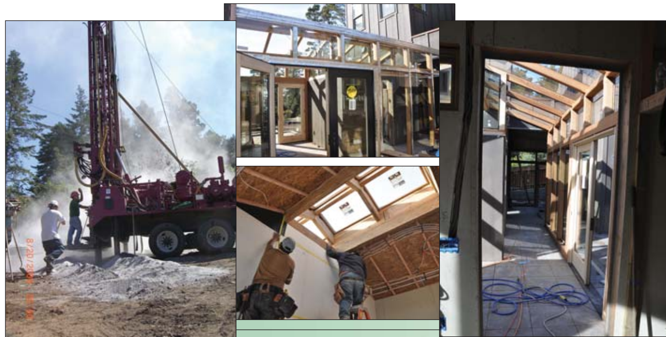
Weeks Drilling Geothermal Rig, Lindal Vestibule Walkway, Serious Materials QuietRock® Drywall, Oregon Shepherd Wool Insulation, Northeast Views
